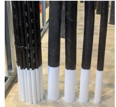
Typical sample of penetrating services with annular gap widths between 10 and 20mm
