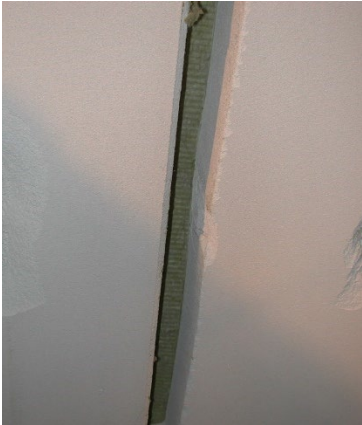
Typical sample of a linear seal in a floor with gap widths below 30mm
